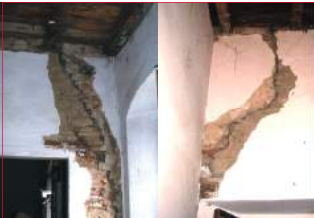
FIGURE 15,16 Cracks due to façade overturning
