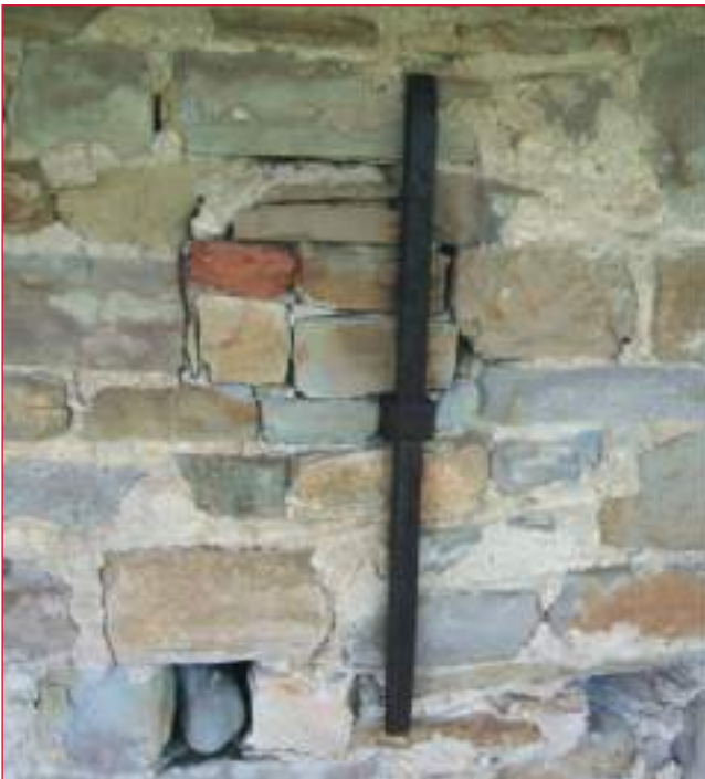
FIGURE 25 Tie rod inserted in breach after the 1869 Vergato earthquake
