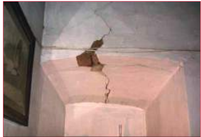
FIGURE 18 Damage to architrave
