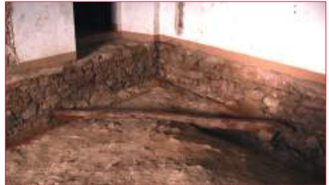
FIGURE 29 Wooden beams to bending walls corner at the extrados of a pavilion vault
