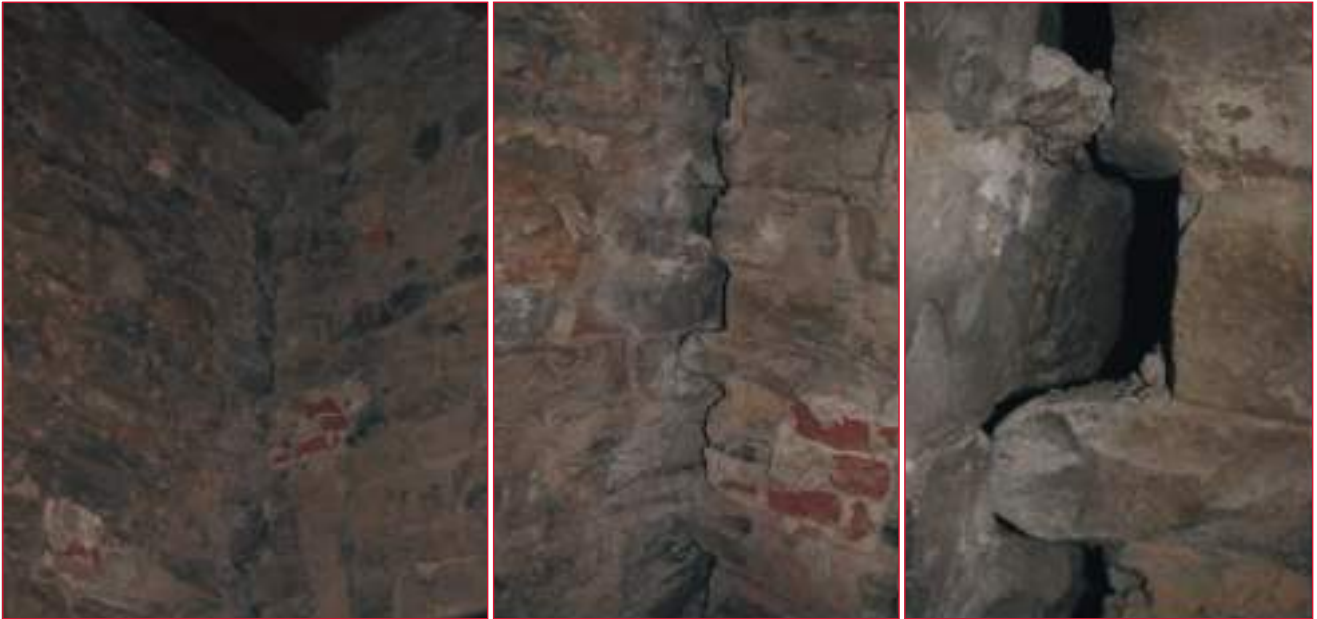
FIGURE 22,23,24 Walls detachment ascribable to 1869 Vergato earthquake
