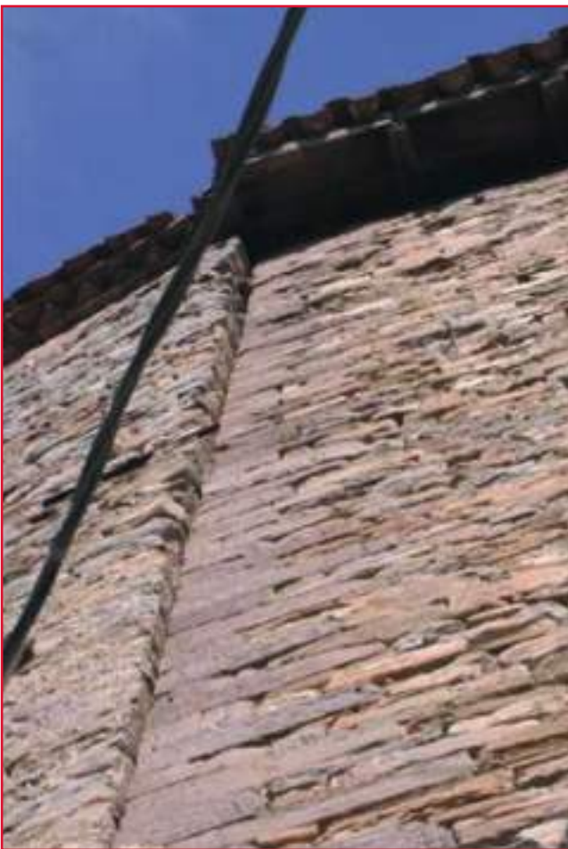
FIGURE 11 Structural discontinuity between adjacent building parts
