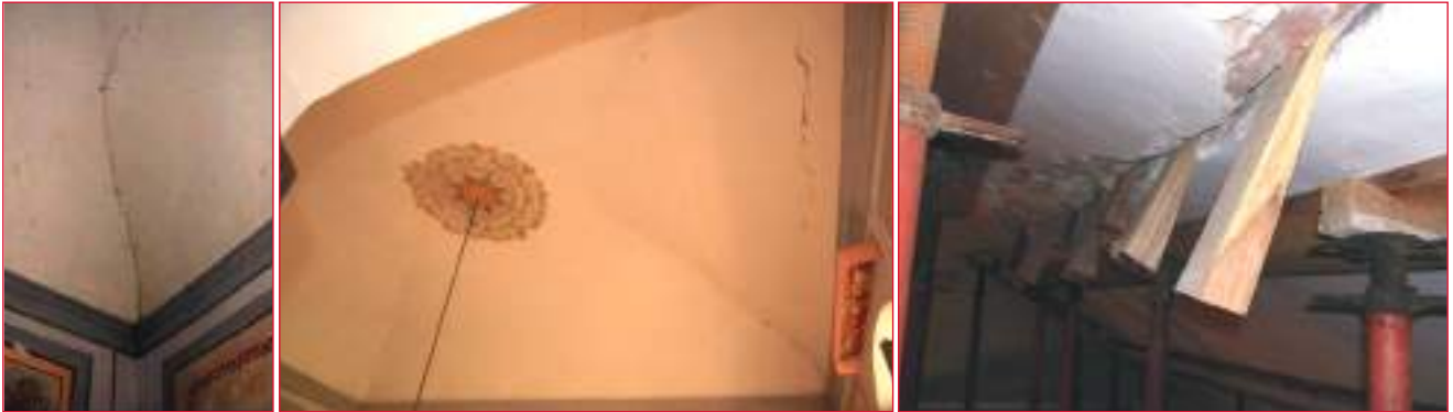
FIGURE 12,13,14 Damage to pavilion vaults
